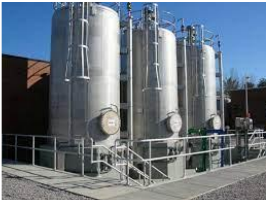
Figure 27: Above ground methanol storage tank | Source: Methanol Institute (2023)
