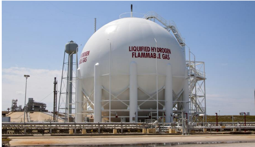
Figure 28: Liquid hydrogen storage vessel | Source: National Aeronautics and Space Administration (2015)
