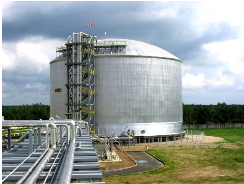
Figure 26: 15,000 tonne liquid ammonia tank | Source: thyssenkrupp Uhde
