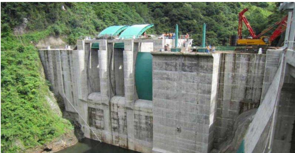
Funded largely by China Development Bank, the $150 million Nadarivatu hydroelectric plant will be operated by the Fiji Electricity Authority (FEA) (Image: HydroWorld)
