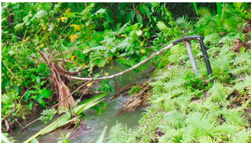
Manakwai, WC repair and improvement over Manakwai river (after pipe was destroyed by flood) (Photo credits: [Kolosori] C Benjamin; [Sumate & Manakwai] M Love)
